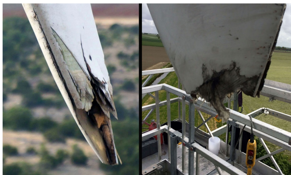
Figure 7. Typical images of wind turbine blade tip detachment, caused by lightning strikes.
