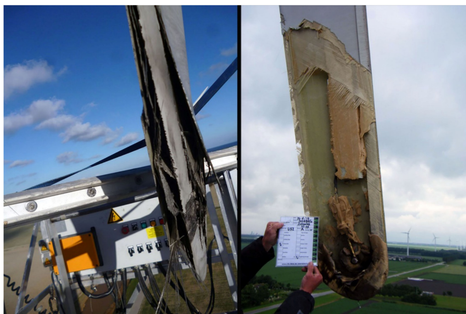
Figure 6. Images of wind turbine blade shell detachment.
