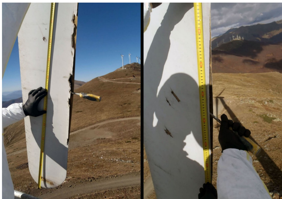
Figure 5. Shell debonding of around 1 m length, starting at 40 cm from the blade's tip ( left photo ) and extending 60 cm in length ( right photo ).
